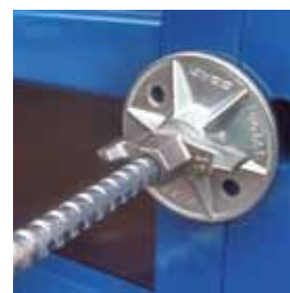
Form-tie holes: only 2 form ties for pouring height of 3.0 m
